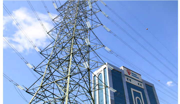
► Tenaga Nasional's transmission tower
